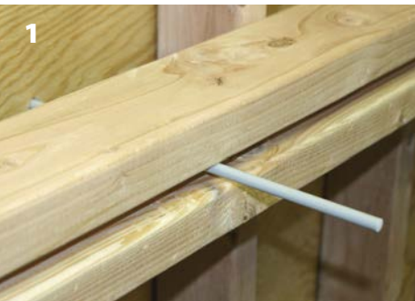
Slide the fiberglass rod through the form. Short lengths of fiberglass rod can be used as internal spreaders; these spreaders can be either tied to the rebar cage, or attached to the tie rod by using two Spreader Clips.
