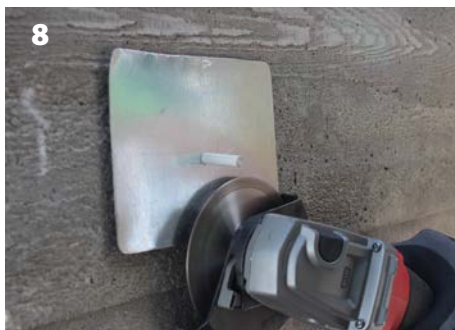
Grind the stubs of fiberglass rod off flush to the concrete structure using a grinder with a diamond blade.
