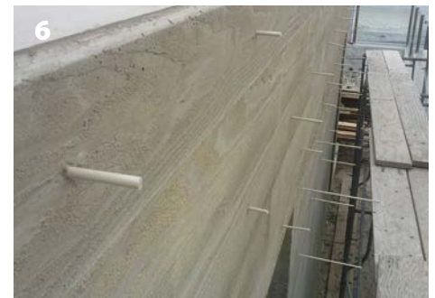
After removing the forms, you will see short lengths of fiberglass rod sticking out of your structure.
