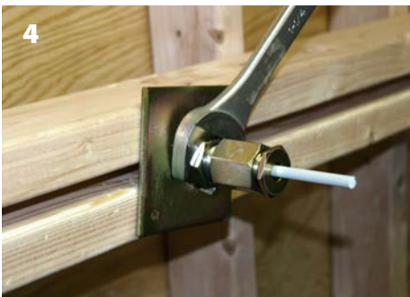
Use the "tensioning nut" to adjust width of form, or tighten form against internal spreaders (there is a maximum of 1/2" of adjustability for each Gripper). You are now ready to place concrete.
