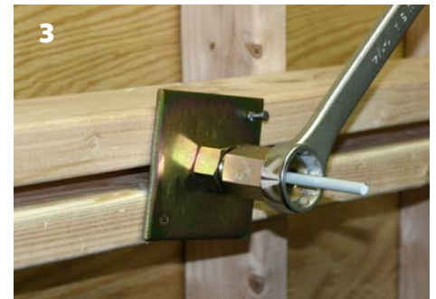
Lock the Gripper onto the fiberglass rod by hand tightening the "tightening bolt," and then with a wrench, a 3/4 turn clockwise. On the opposite side of the form, lock another Gripper onto the fiberglass rod.
