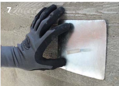
7 To ensure protection of exposed concrete surface, drill a hole slightly larger than rod diameter in a piece of sheet metal, slide over rod, then cut.
