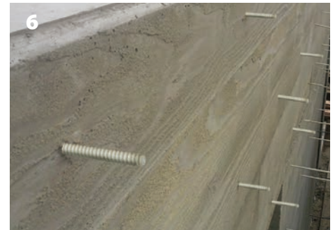
6 After removing the forms, you will see short lengths of fiberglass rod sticking out of your structure.
