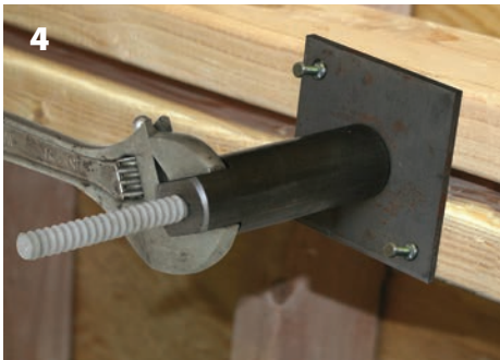
4 On the opposite side of the form, lock another Form Fixture onto the fiberglass rod.
