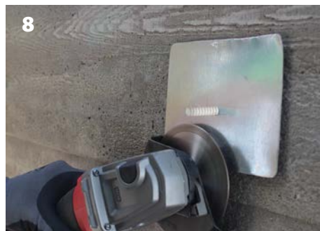
8 Grind the stubs of fiberglass rod off flush to the concrete structure using a grinder with a diamond blade.
