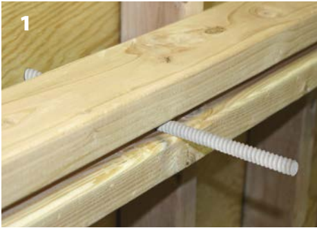
1 Slide the fiberglass rod through the form. Short lengths of fiberglass rod can be used as internal spreaders; these spreaders can be either tied to the rebar cage, or attached to the tie rod by using two Spreader Clips.
